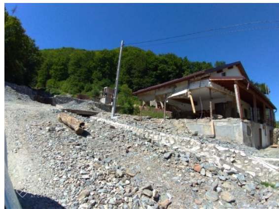
Fig. 1.2. House destroyed as a result of the torrential transport - Rucăr locality
