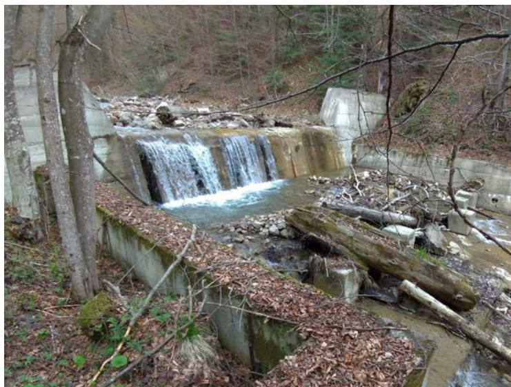
Fig. 5.40. Apron silting Structure 11 B 2,0 –Tesla Creek
