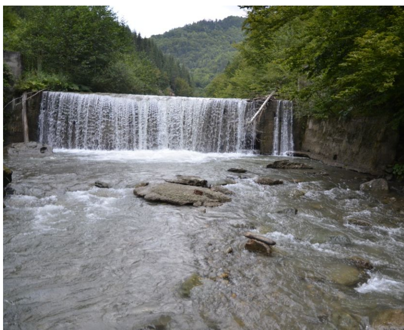
Fig. 5.34. Total apron detachment at structure 3 B 4.0 - Repedea Valley
