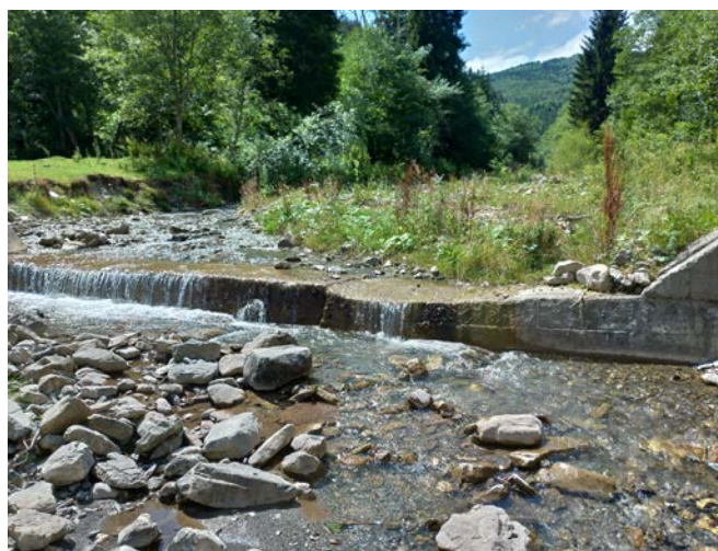
Fig. 5.28. Vertical crack that generated the rupture of the spilled area of the structure 9 B 0 – Tigăi Valley
