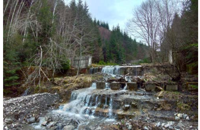
Fig. 5.38. Detachment recorded at the terminal spur Structure 2 B 3,0 –Nanului Creek
