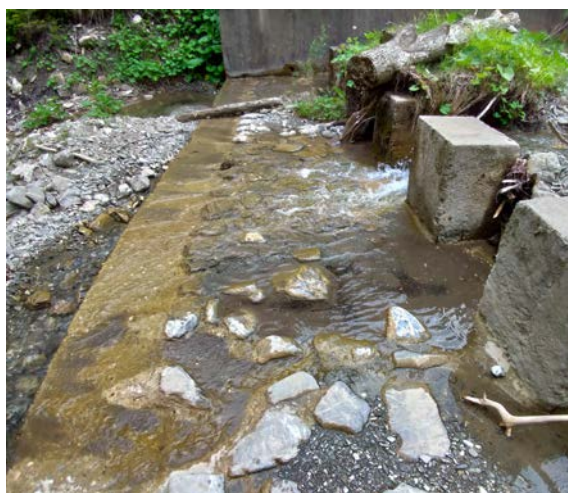
Fig. 5.37. Apron erosion at 11 B 2,0 structure - Tigăi Valey (Foto: Mihalache, 2020)
