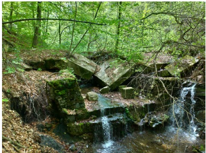
Fig. 2.2. Overturning and breaking of the body of the structure after torrential flow of August 31, 1085
